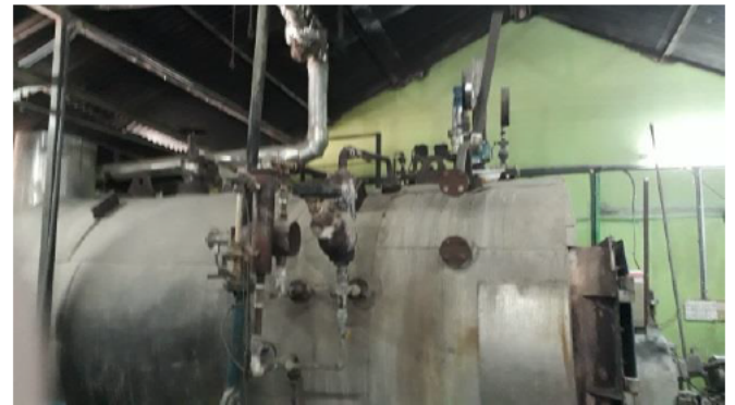
A boiler can be dangerous, if it is not run properly:
